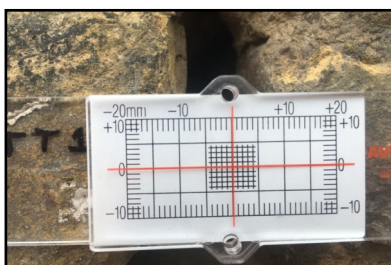
Tell Tale Crack Gauge
